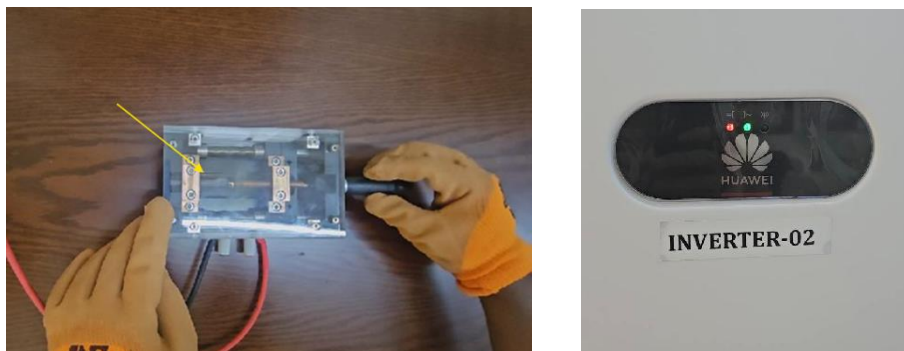
Figure: Arc generating from the Arc generator and inverter alarm LED blinking
