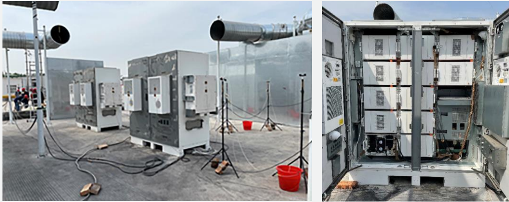
Figure 17. Multiple observation devices used to accurately capture test results Left: test site layout; Right: tested cabinet
