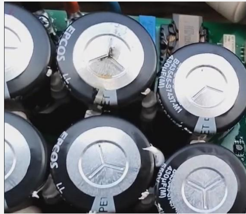
Damaged Bus capacitor
