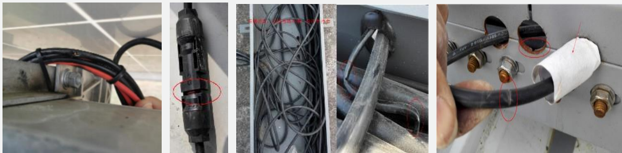
Cables tied to a support
