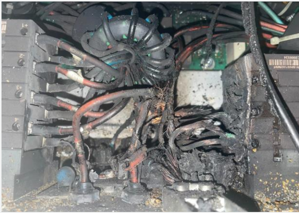
Burned DC cables
