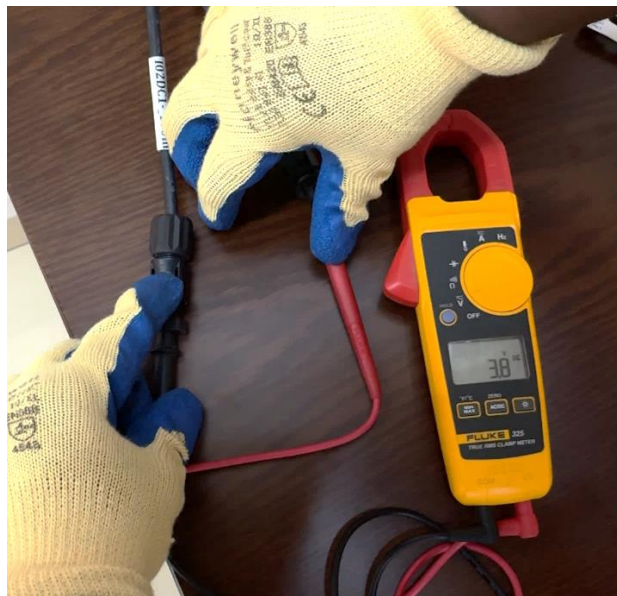
Figure: After AC switch turned off the string voltage is 3.8V DC (>30V DC)
