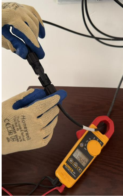
Figure: PV+ and PV- is shorted after remote shutdown
