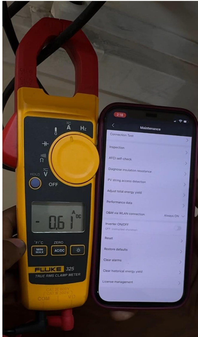
Figure: All string current is 0.61A DC after remote shutdown
